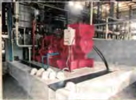
Steam turbine at the production facility
